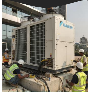
Air Cooled Chiller
