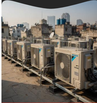
VRV System Installation
